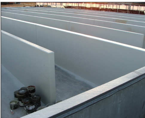
Various concrete structures at the Central Water Reclamation Facility in Pensacola, FL were topcoated with Series 436 Perma-Shield FR to provide protection against abrasion and chemical contact.
