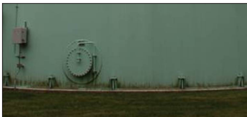
The top two photos show the mold and mildew growing on the Wadsworth standpipe when coated with an acrylic polyurethane system. The bottom photo shows very minor mildew growth due to grass clippings, after a Tnemec fluoropolymer system was applied.
