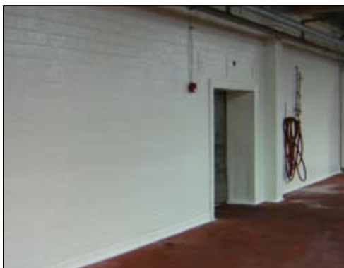
Before and after photos of the walls at the Smithfield Foods plant in Landover, MD. Now protected with a Stranlok fiberglass-reinforced coating system, the walls can withstand thermal shock from daily high-pressure steam cleaning.
