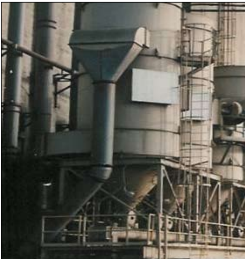
A zinc/epoxy/urethane coating system has been protecting the dust collectors at the Bunge Grain facility in Destrehan, LA since 1984 with no signs of rust.
