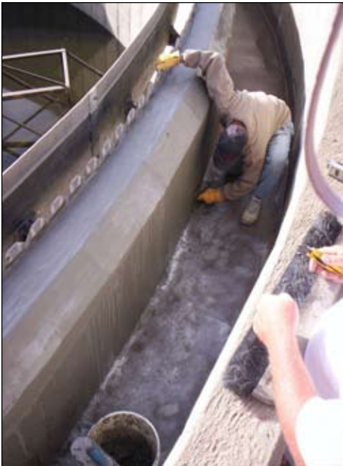
Tnemec's Perma-Shield System featuring Series 435 Perma-Glaze protects the clarifiers at the Brighton WWTP from biogenic sulfide corrosion.
