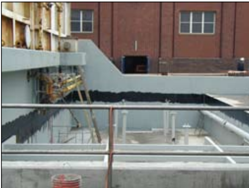
Tnemec high performance coatings protect steel and concrete surfaces within the secondary containment area at the Detroit, MI Wastewater Treatment Plant.
