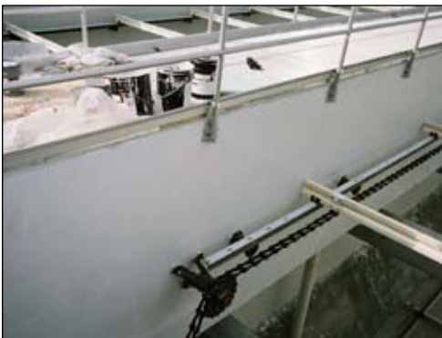
Series 215 Surfacing Epoxy was applied as a full skim coat to smooth out the entire wall and fill surface imperfections in the existing concrete troughs at the Cedar Creek Water Treatment Plant in Winder, GA.
