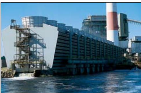
Bottom photo: This cooling tower was constructed and coated in 1989 after Hurricane Hugo destroyed the existing cooling tower. The owner wanted a proven coating system to extend service life and eliminate shutdowns. Three coats of Tnemec epoxy were applied to the interior and exterior by Dunlap, Inc., of Greenville, SC. (Coating system: 66/66/66)
