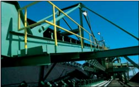
Top two photos: The conveyors and stacker/recycler at William Station were painted in 1987 by Hames Contracting of Columbia, SC. The Tnemec MCU primer and Endura-Shield coating are still performing as verified by a 2007 site visit. (Coating system: 530/27/73)
