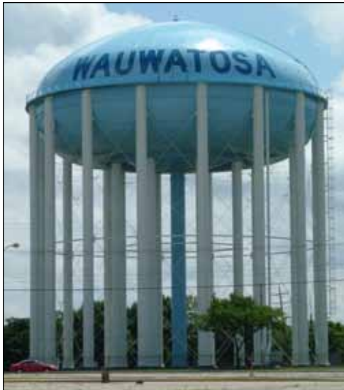
Before and after photos of the 2.5 Million Gallon Torosphere in Wauwatosa, WI. The interior was repainted with Tnemec protective coatings in 1998 and the exterior, as shown above, was repainted in 2001.
