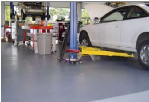
The service area floor at Dene Lambkin Hyundai in Quincy, IL features a coating system from Tnemec's StrataShield flooring line.
