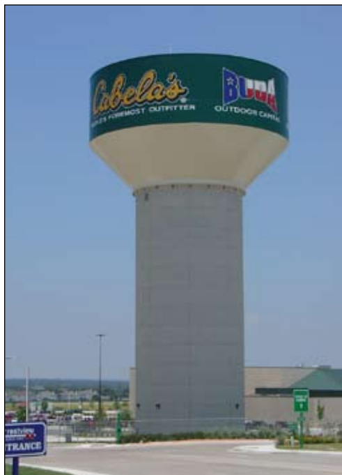
Series 700 HydroFlon, a fluoropolymer polyurethane finish coat, protects the exterior of the Cabela's water tank in Buda, TX, while Series 141 Pota-Pox 80, a high-solids polyamine epoxy, protects the interior.
