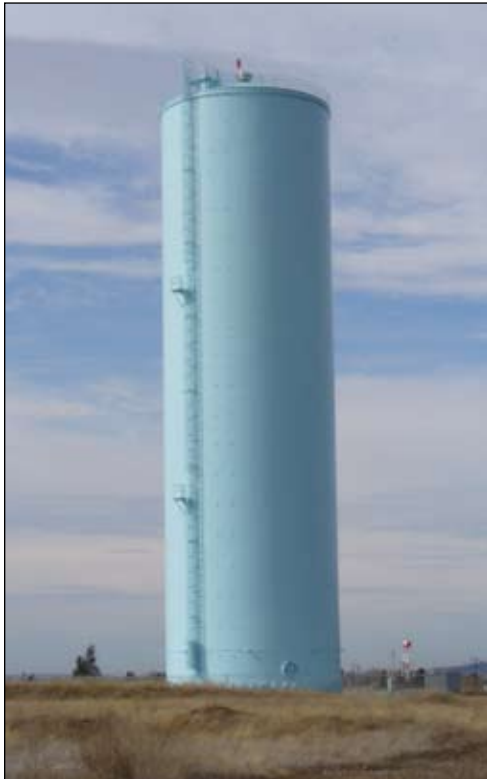
Both the interior and exterior steel of this standpipe in Post Falls, ID, are primed with Series 91-H 2 O Hydro-Zinc, the first organic zinc-rich primer to be ANSI/NSF Std. 61 certified for use in potable water.
