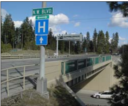
Tnemec's Omnithane, a moisture-cured urethane containing MIO and zinc, was used to protect the Northwest Boulevard Bridge in Coeur d'Alene, ID, a popular tourist destination.
