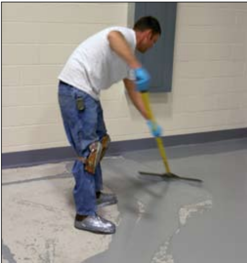
Series 245 Ultra-Tread S, a polyurethane modified concrete floor topping, provides a durable coating system that withstands thermal shock and chemicals used in the decontamination process at the UniTech Services Group Building in Morris, IL.
