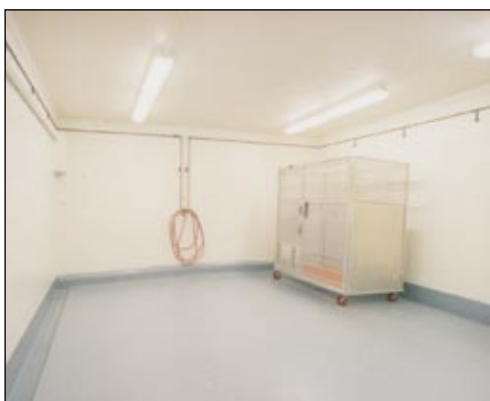
The floors and walls at The University of Missouri College of Veterinary Medicine's animal holding center are protected with Tnemec's StrataShield line of coatings.
