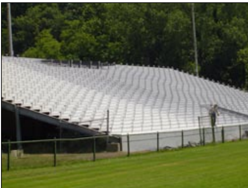
The Dormont Memorial (top) and Valley Senior High School Memorial (bottom) Stadiums, both located in Pennsylvania, are protected with Tnemec high-performance coatings.
