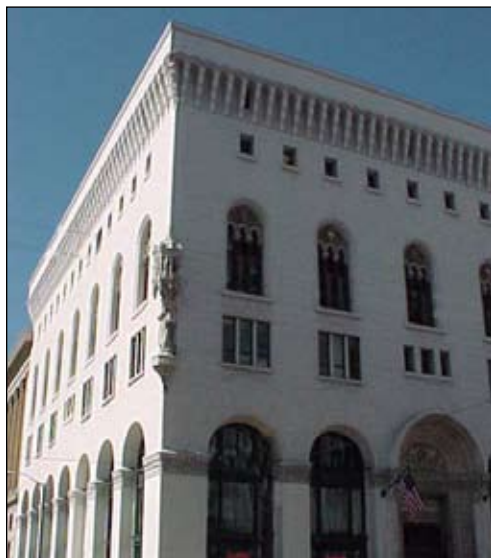
The exterior of the building at 25 Van Ness Avenue in San Francisco, CA is protected with various Tnemec masonry coatings including Series 156 Enviro-Crete, a breathable waterborne acrylate coating.
